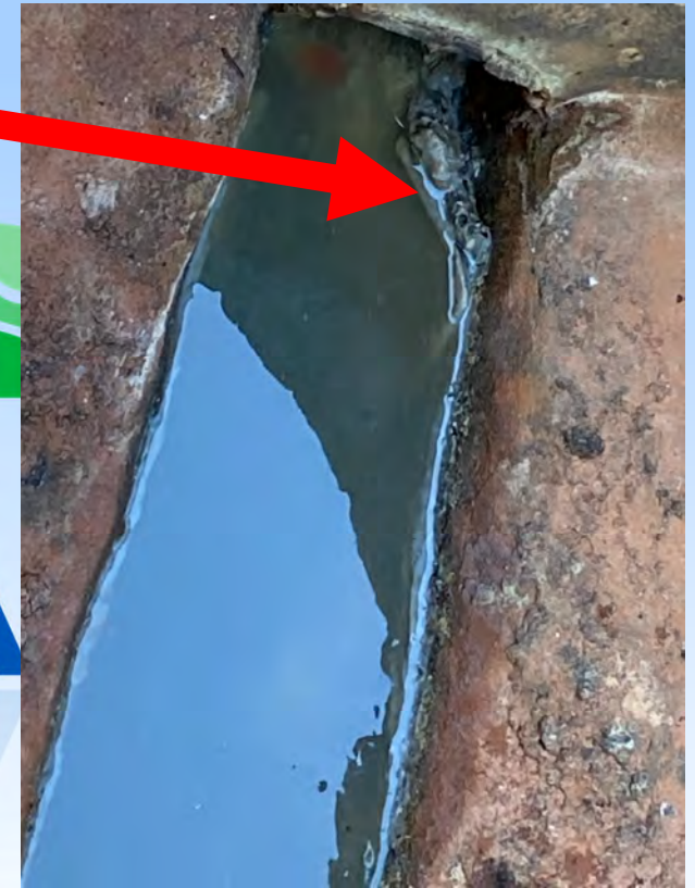
Grease build up on an OJRSA line that was "jetted" from a Member City line into the trunk sewer (October 2023)
