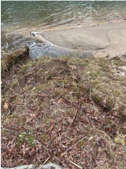
Photopoint 18: 34.69119, -83.15472 Erosion can likely be attributed to the mismanagement of the riparian buffer.
