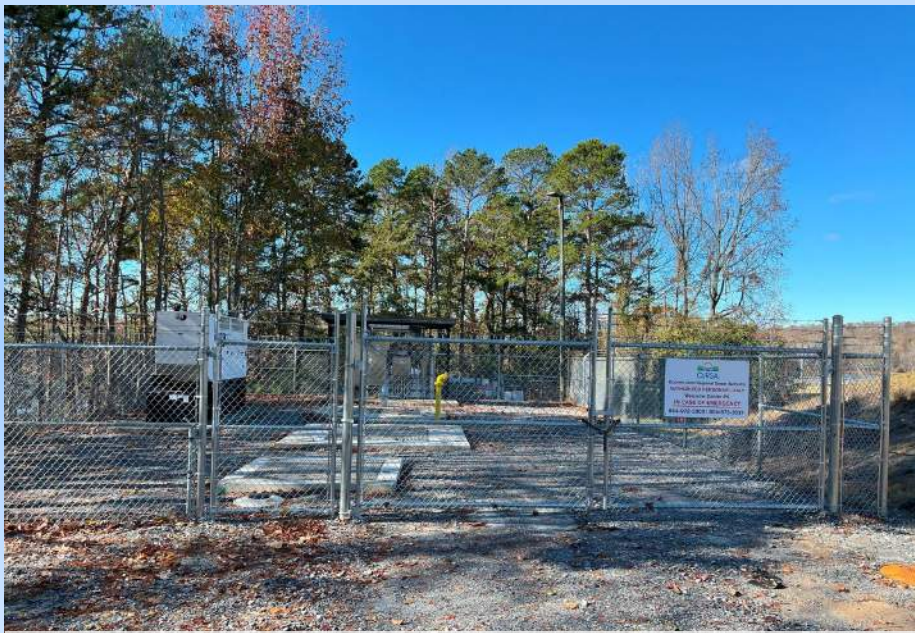
I-85 Phase II: Welcome Center Pump Station
