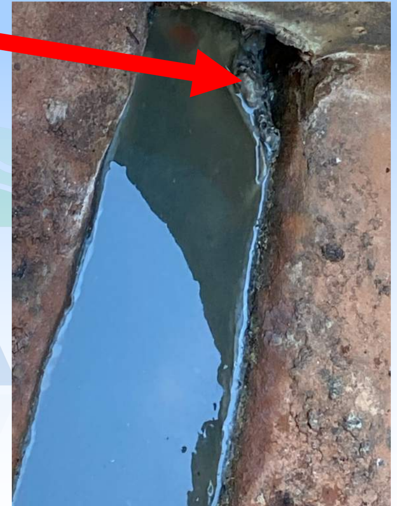
Grease build up on an OJRSA line that was "jetted" from a Member City line into the trunk sewer
