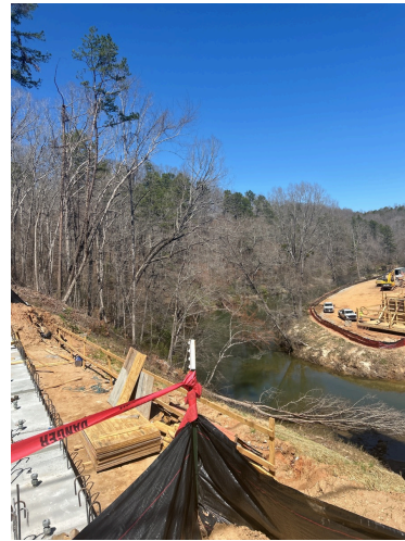
Photopoint 03: 34.68535, -83.15196 View of bridge construction project along Chauga River. Note silt fencing along the banks of the river.
