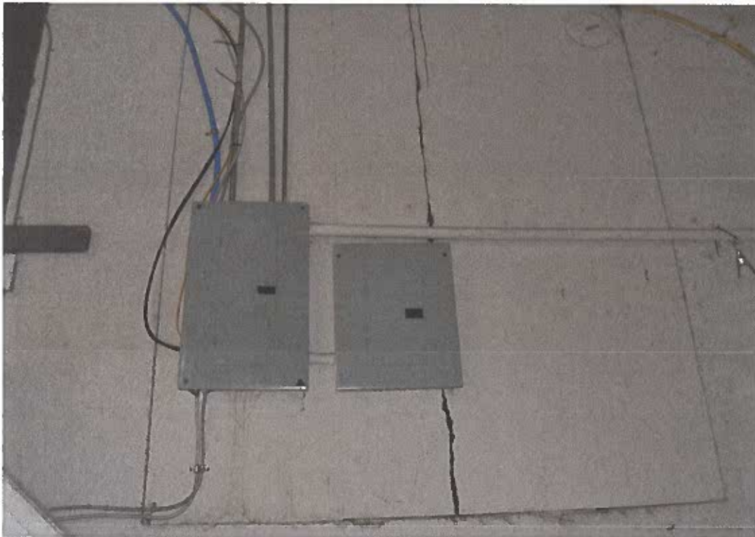
Close-up View of Existing 100 AMP Electrical Service to be Upgraded.
