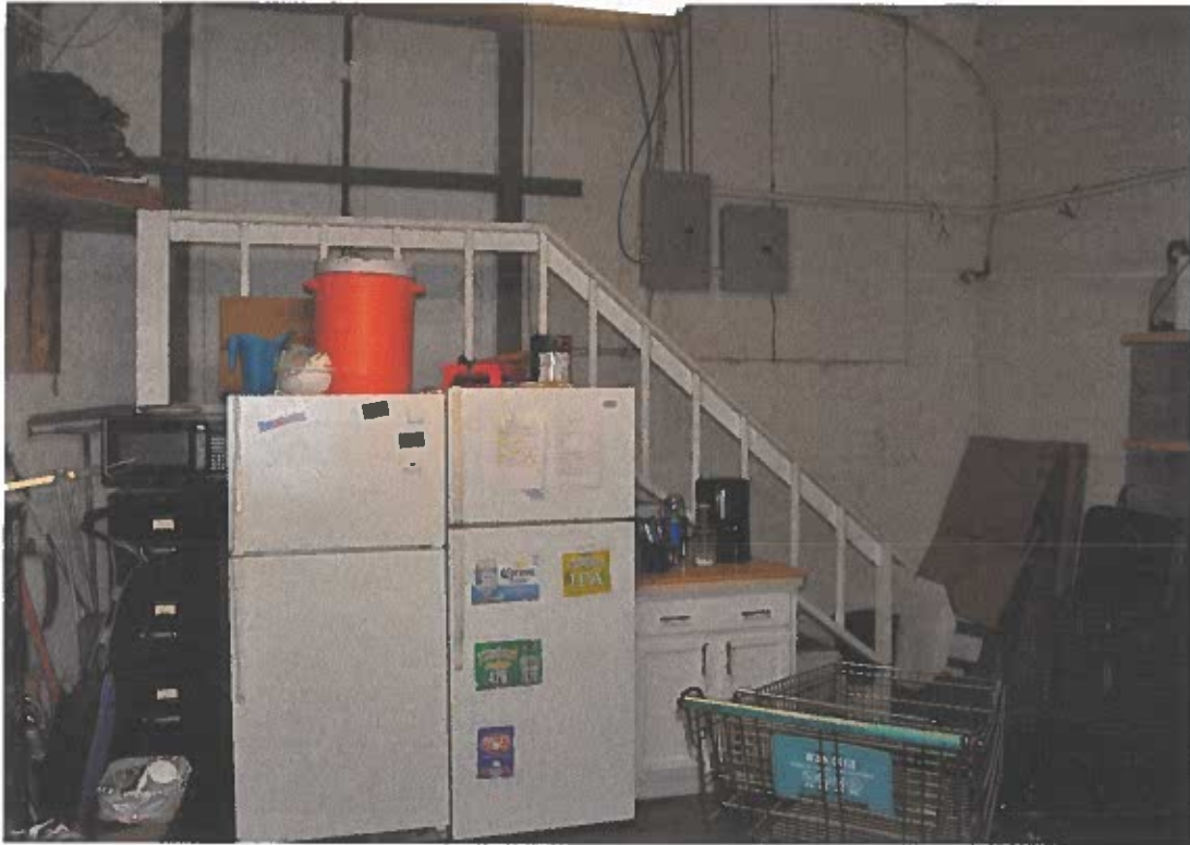
View of Existing Electrical Service on Rear Wall of Subject Unit.
