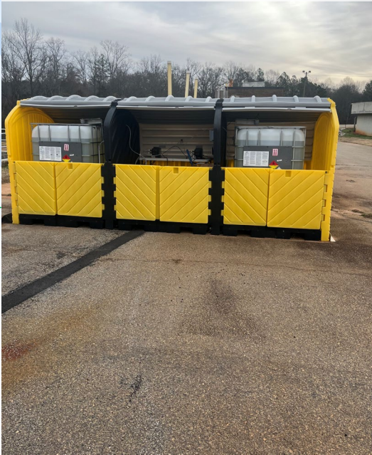
Peracetic acid disinfection system
