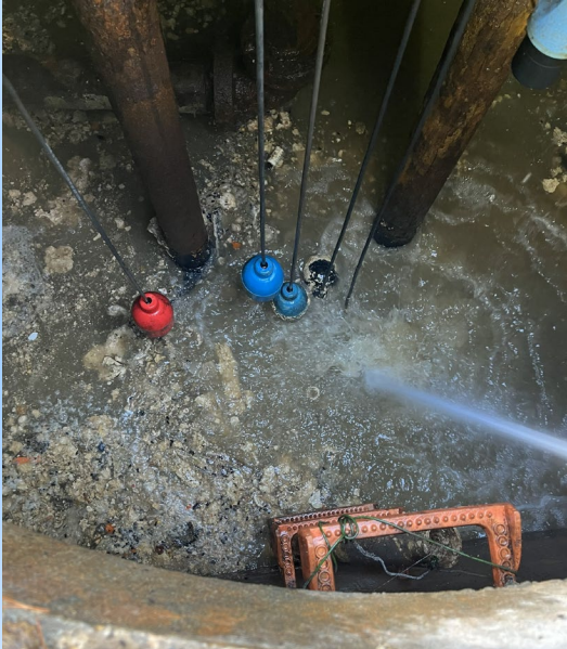
Choestoea PS wet well before cleanout...
