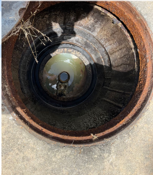
Effluent chamber in FOG device...what it SHOULD look like
