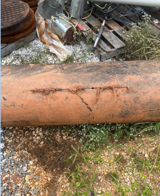
Crack on Perkins PS force main
