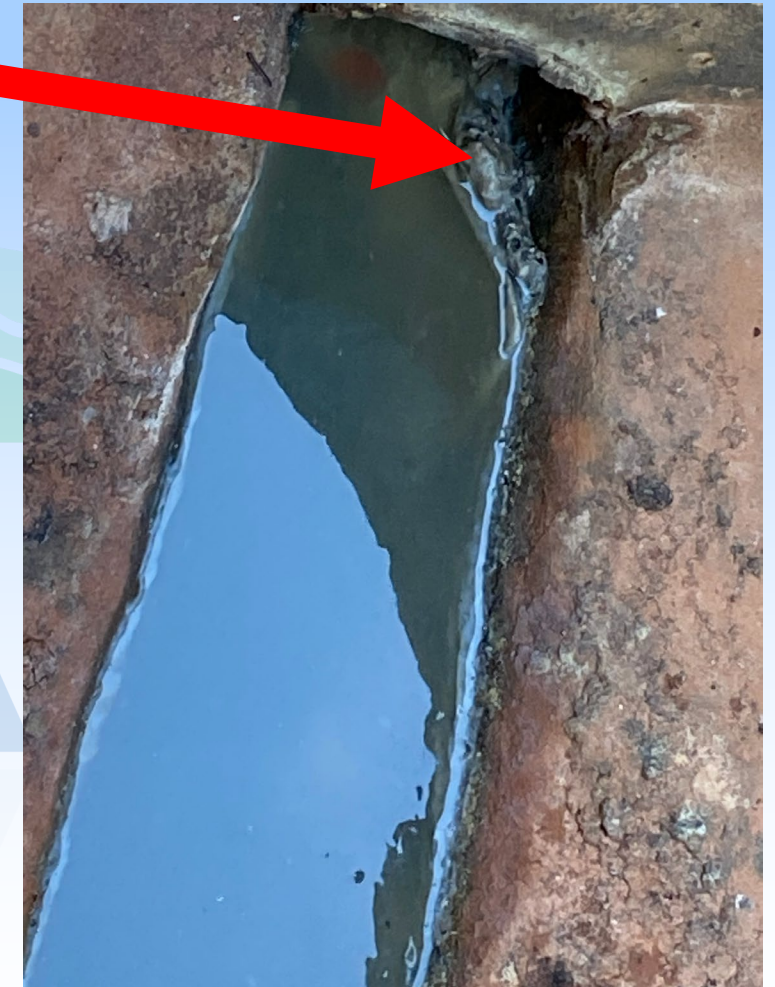
Grease build up on an OJRSA line that was "jetted" from a Member City line into the OJRSA trunk sewer
