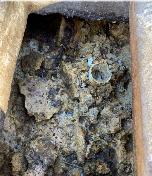
FOG control device...what it SHOULD NOT look like
