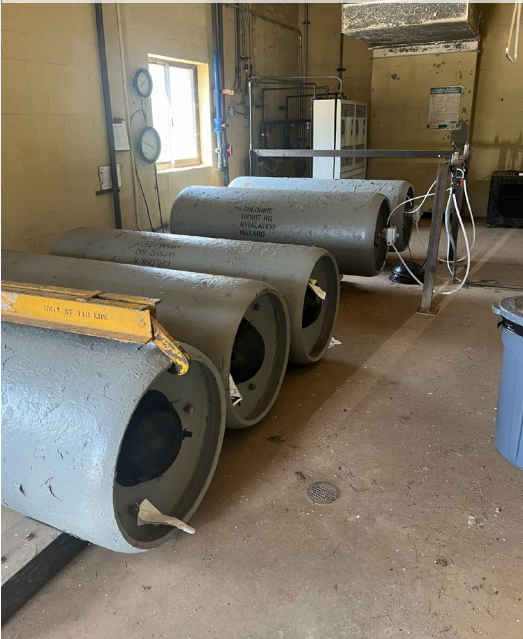
Chlorine gas disinfection system
