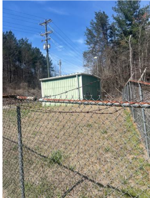
Photopoint 02: 34.68678, -83.15666 Pump station adjacent to Highway 76.
